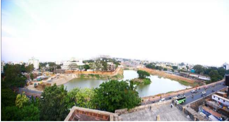
Establishment of Sports Fishing cum Eco Park at Chetpet, Chennai ongoing work at a total cost of Rs 42 crore
